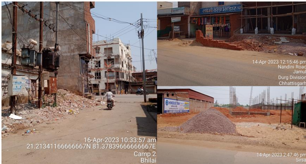
Figure 3.26: Construction material and debris near construction sites
